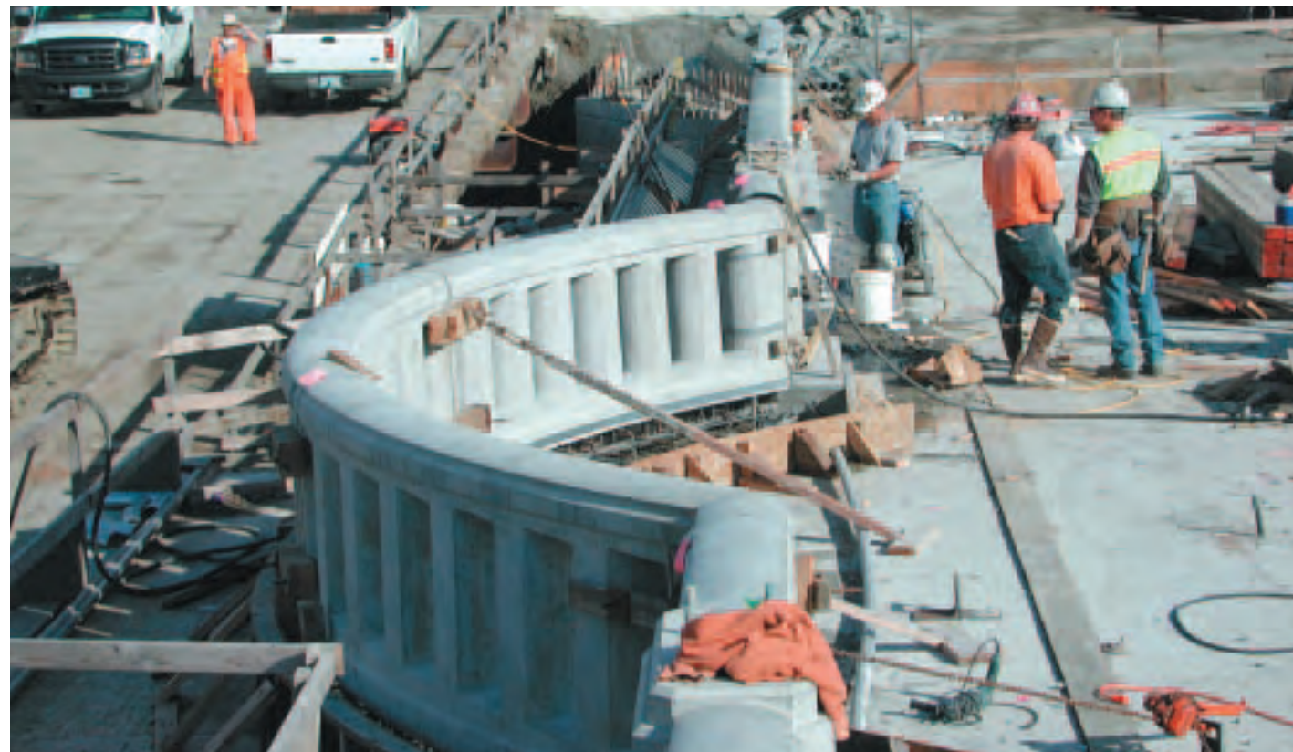
INSTALLATION OF THE RAILING ON THE OLYMPIA-YASHIRO FRIENDSHIP BRIDGE PROGRESSED MUCH QUICKER AFTER SWITCHING TO PRECAST CONCRETE.
